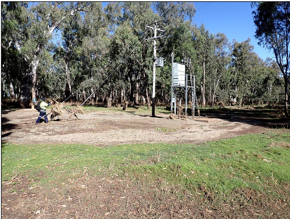
Plate 4: Flood debris entangled in electrical infrastructure at existing bore location.
