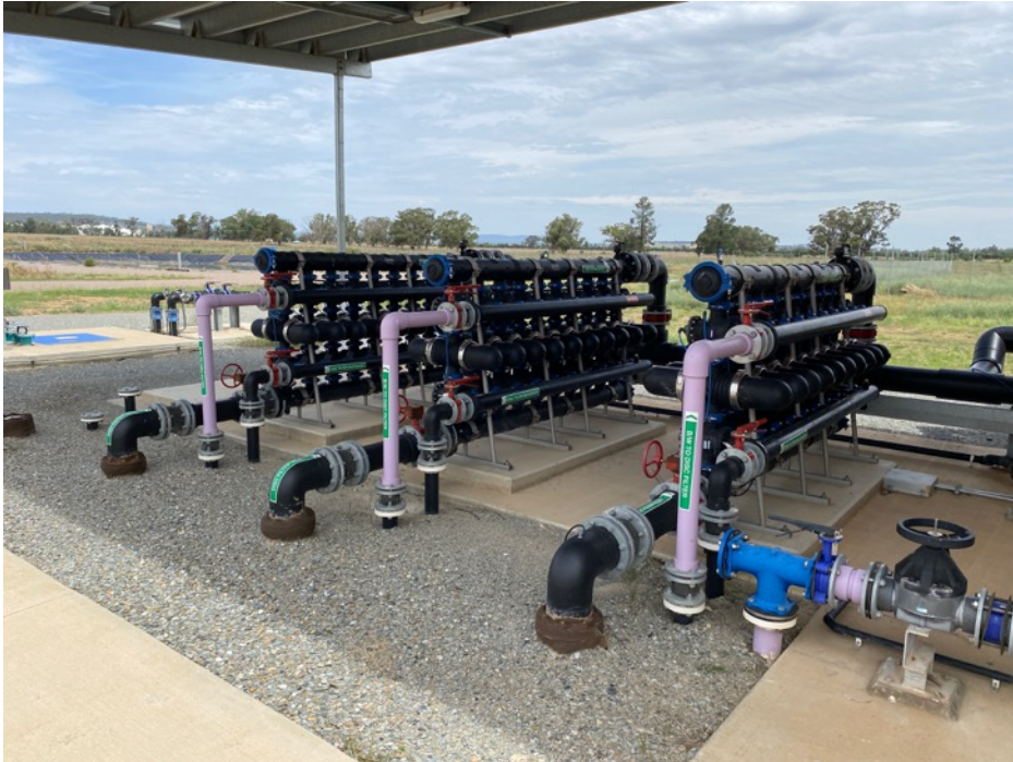
Figure 4-30: Advanced Water Recycling Facility - membrane filters
