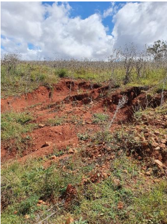
Plate 5 Erosion and previous excavation at the existing dam
