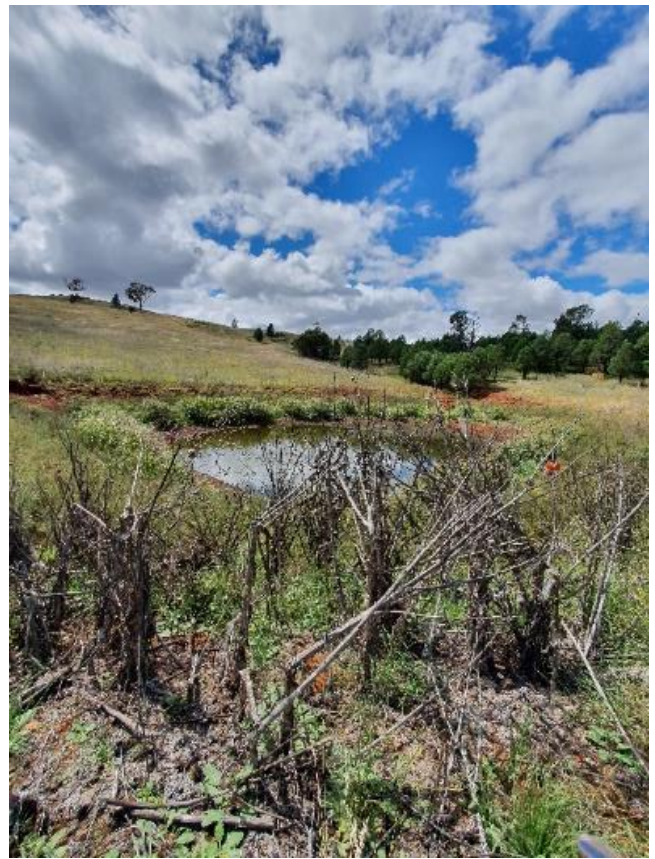
Plate 4 Existing dam with degraded fringing vegetation and eroding banks
